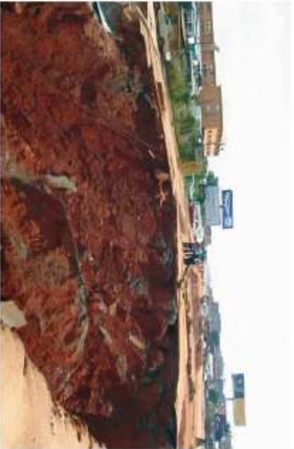
Figure 5.3: Mass movement affecting express highway in Onecha City, Nigeria, which is associated with gully erosion development.
